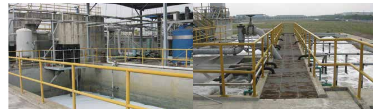
Waster water treatment of the factories
